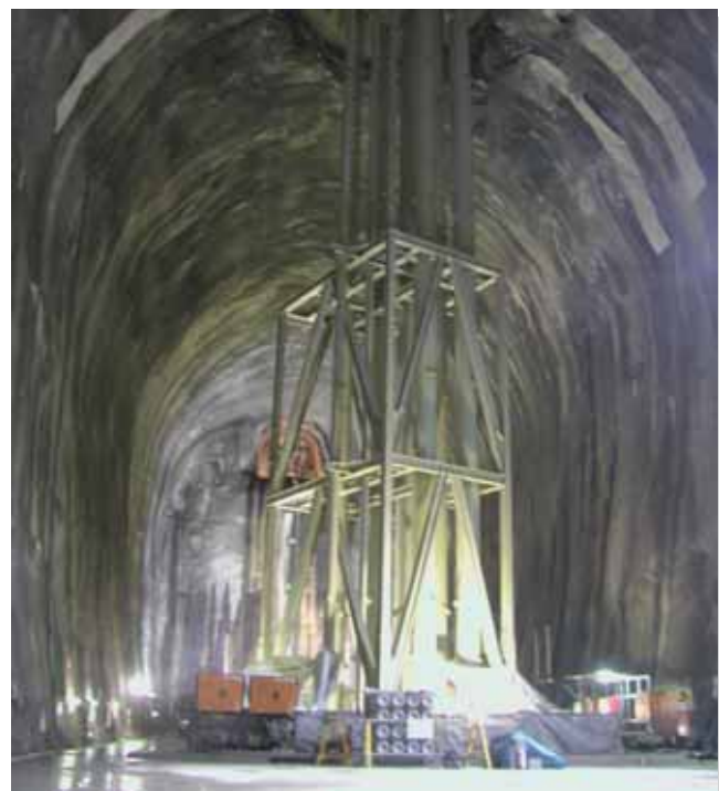
Special Account for Energy Policy/National Stockpiling Project/ Kurashiki National LP Gas Stockpiling Base/Kurashiki City, Okayama Prefecture
